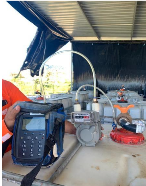
Figure 5 - Measurement of gas flow and composition in the reactors installed at GNR/ASMOC
